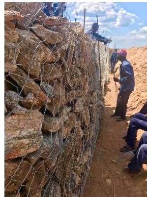
Fig 19A gabion is constructed to provide stability to the trench: Photo: Mariri
