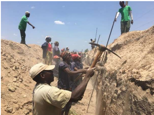
Fig 18 Mbamba community members are digging the elephant and buffalo safe trench. Photo: Mariri
